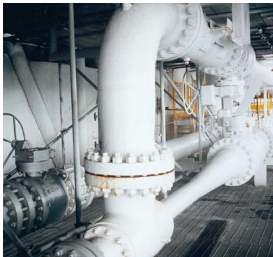
WELLCOM Gas system installed on Hewett
